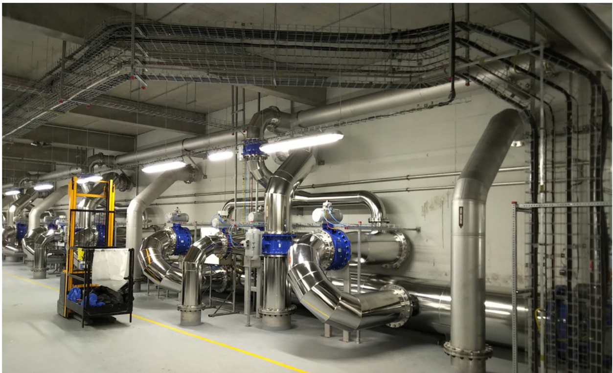
Technological background of the engine room.
