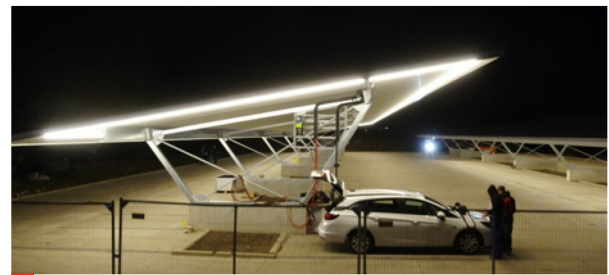
PV charging stations.
